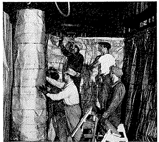
Here an efficient crew of Santa Fe workmen are deftly applying blanket form insulation inside a refrigerator car in for general repairs at the West Wichita, Kan., shops.
